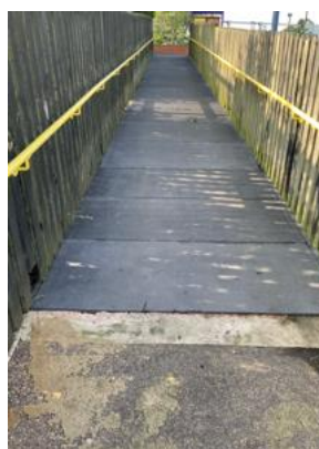
Ramp surfacing deteriorating
