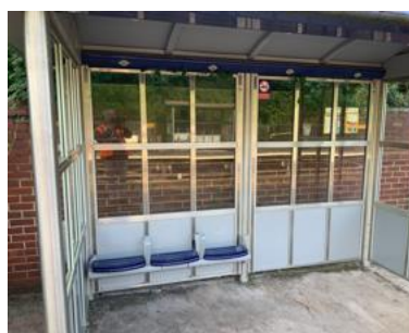
Figure 1: Issues at Goldthorpe rail station
